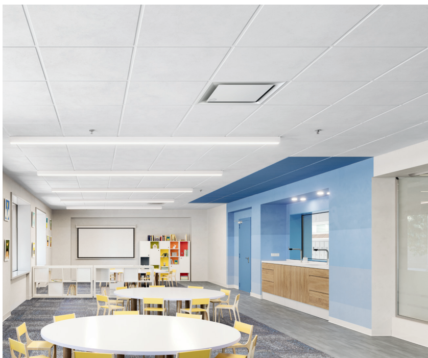
In-ceiling air purification technology draws air up and away from kids sitting at their desks and then recirculates clean air back into the room
